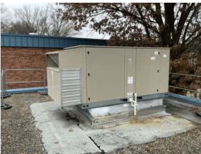
29 - PACKAGED ROOFTOP UNIT
