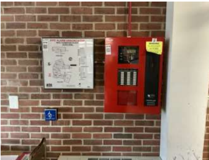
33 - FIRE ALARM PANEL / ANNUNCIATOR
