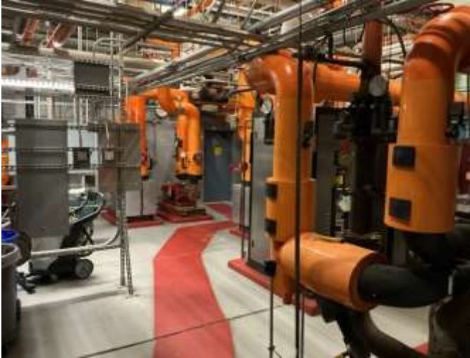
25 - MAIN MECHANICAL ROOM
